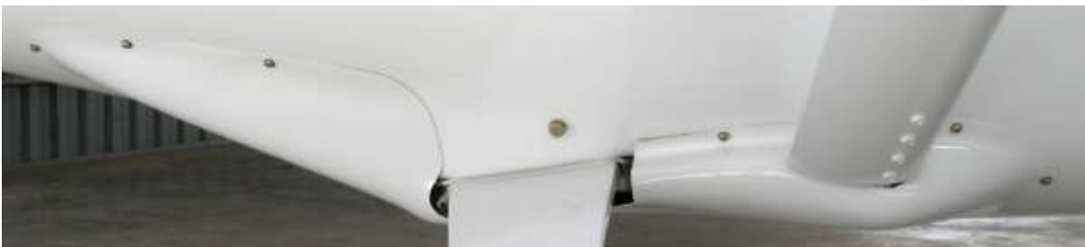
Right hand side strut/main gear fairing from below (top photo) and side on (above)
